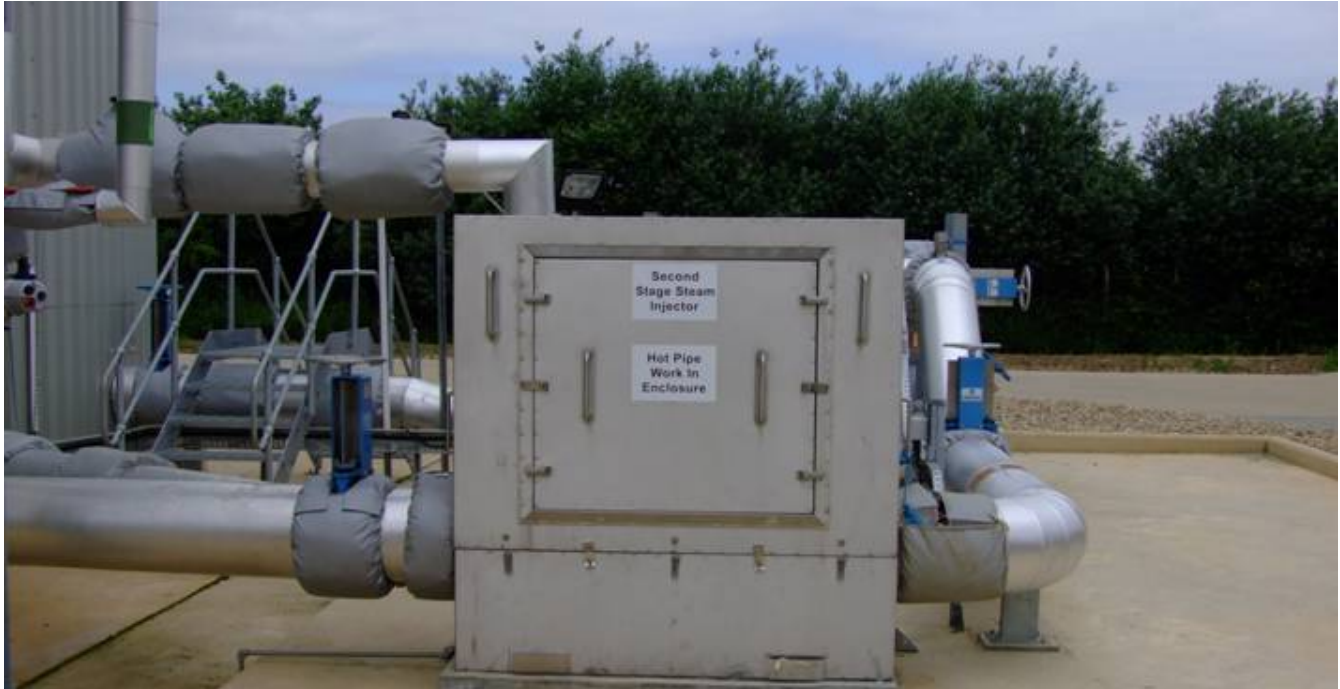
Figure 2: Monsal ADT Re:Smart, Installation
