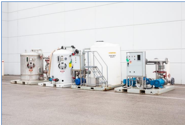
Figure 6: SUEZ proprietary multi vessel water purification system with interstage testing and automation control
